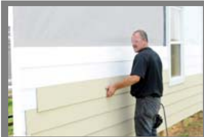
Installing siding on a building frame where exterior insulation has been applied takes special care to make sure the cladding gets properly attached to the frame. (Photo courtesy of Progressive Foam)
